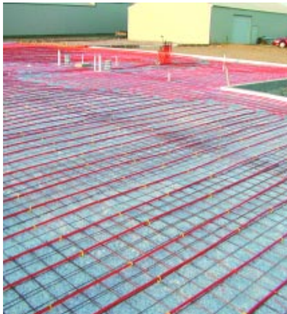
RadiantPEX used in an industrial slab heating system.
