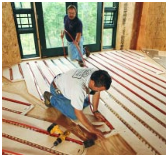
RadiantPEX in a residential SubRay™-heated floor.
