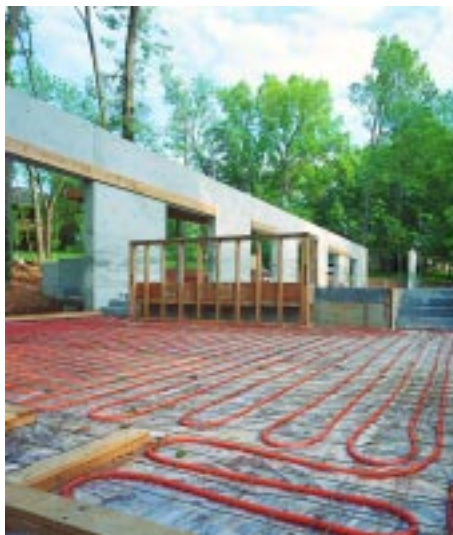
RadiantPEX in a residential slab heating system.
