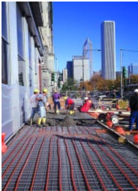
RadiantPEX in a commercial snowmelting system.
